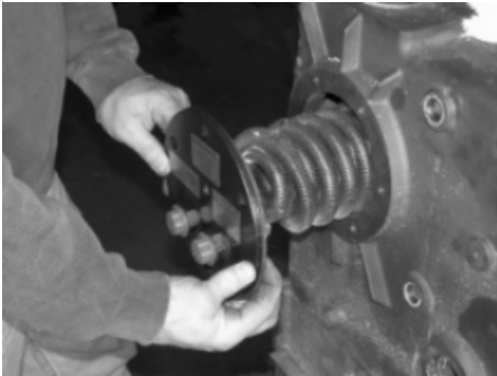
Figure 7: Tankless Heater Installation
